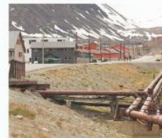
D Overground service pipes
