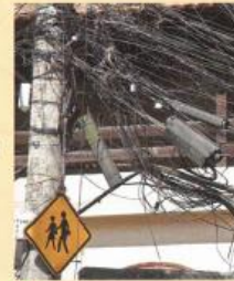
E Illegal electricity connections in a favela
